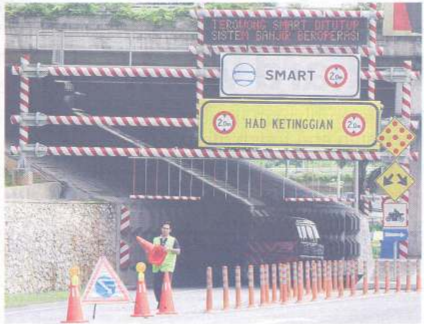
Closed: A worker placing traffic cones in front of the Smart Tunnel to facilitate flood mitigation work.
